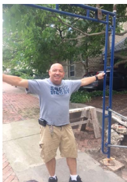
Our Building Manager, Jaime Durango, holds up the final piece of scaffolding to be removed from Meeting House restoration.
